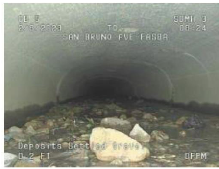
Picture of a Brisbane storm drain, depicting debris that need removal
